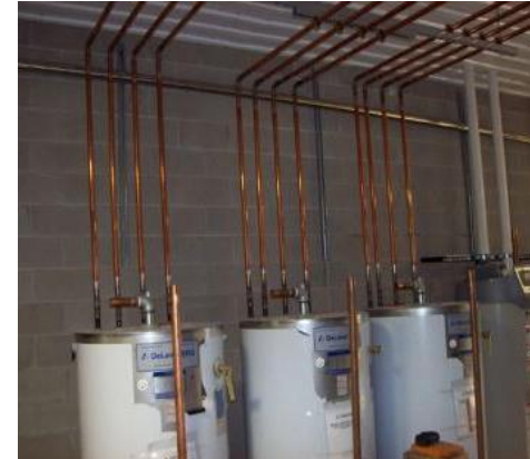
Heat Recovery - Refrigeration Units $0.28 per kWh annual savings
